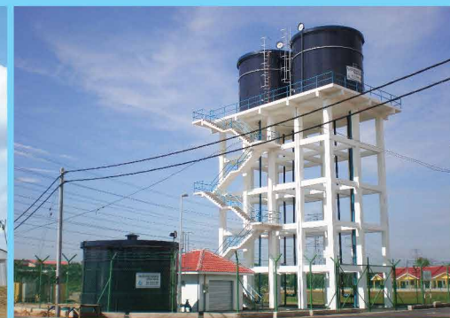
2 x 33,000 gallons & 25,300 gallons Pahang
